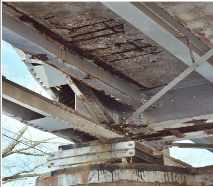
Corrosion of steel & concrete spalling
